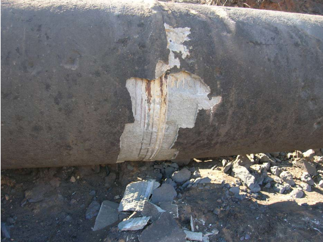
Fig. 6. Fire damage to section of the Sutherland Pipeline, owned by the City of San Diego, as a result of the 2007 Firestorm event in which as many as seven fires burned 369,000 acres or 13% of San Diego County (OES 2008).
